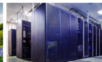
Data center energy backup
