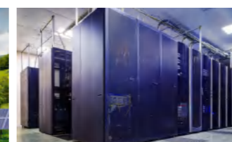
Data center energy backup
